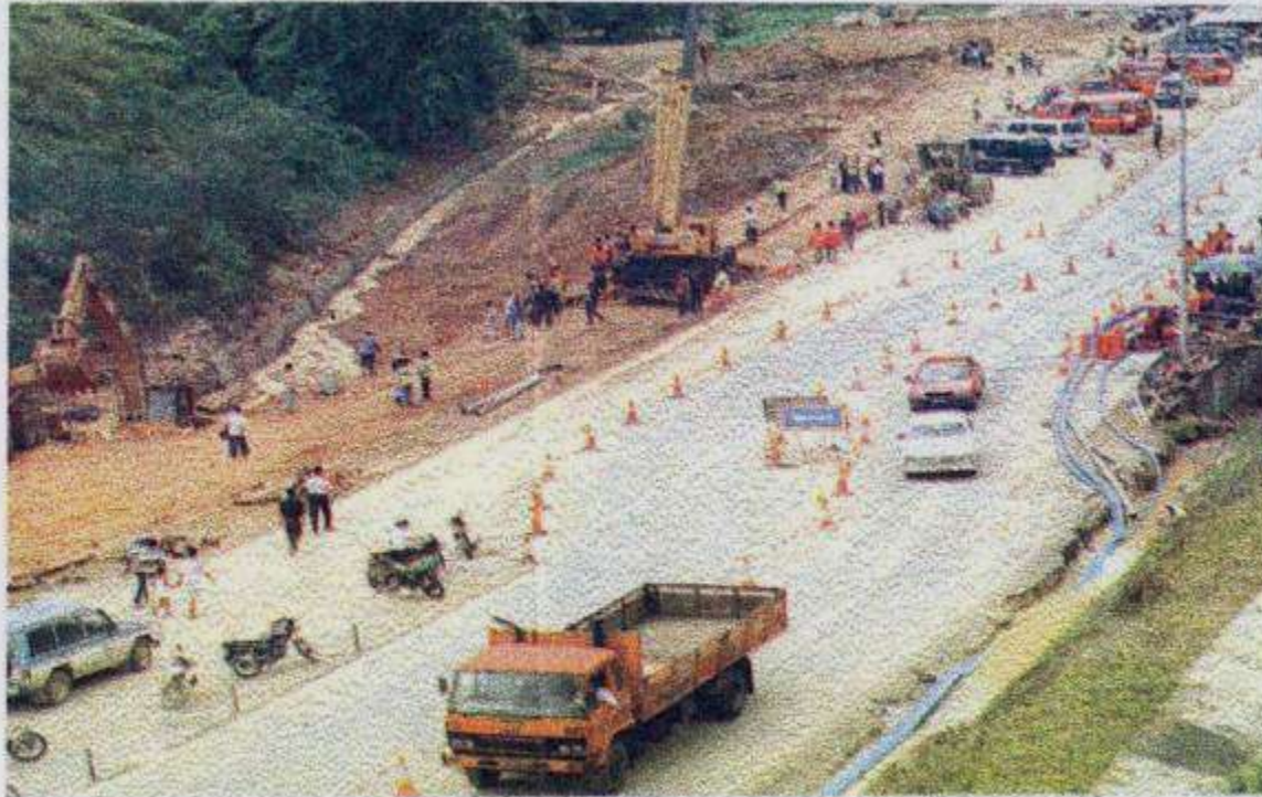
Photo 4 : The scene at the landslide location
